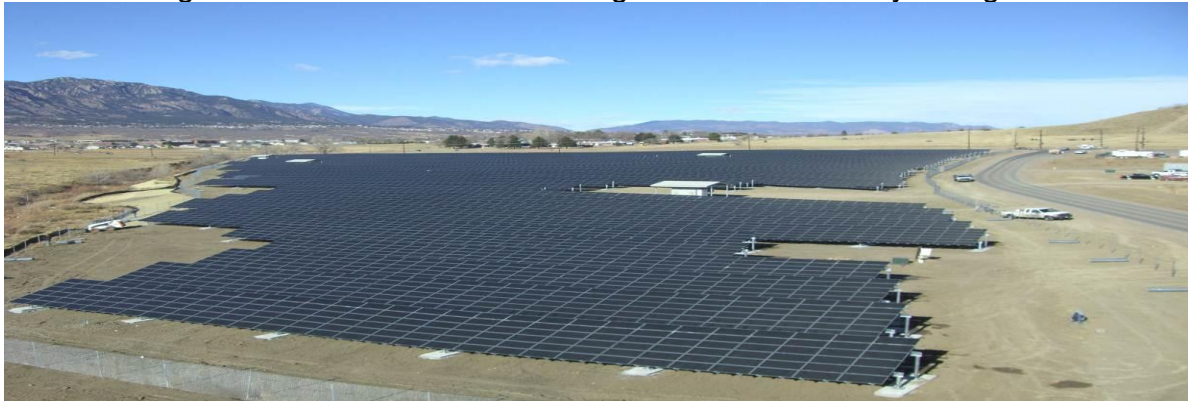
Figure 2. Large scale Solar PV array
