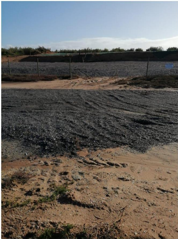
8) Illegal moving of earth
