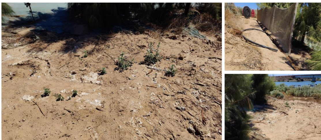
Figure 5.4. Evidence of Sewage leakage observed during site visit.
