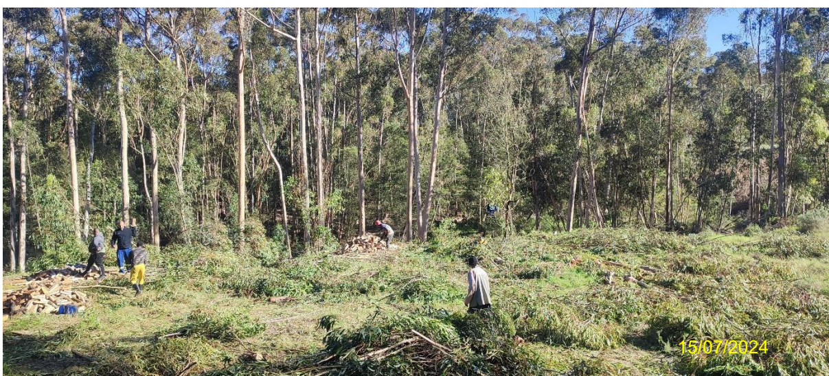
Photo 5: Eucalyptus tree clearing taking place on proposed development site below Bloekombos dam.
