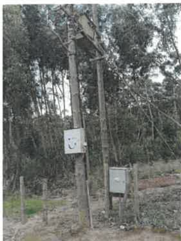
Photo 2: Point of power supply to WTW
