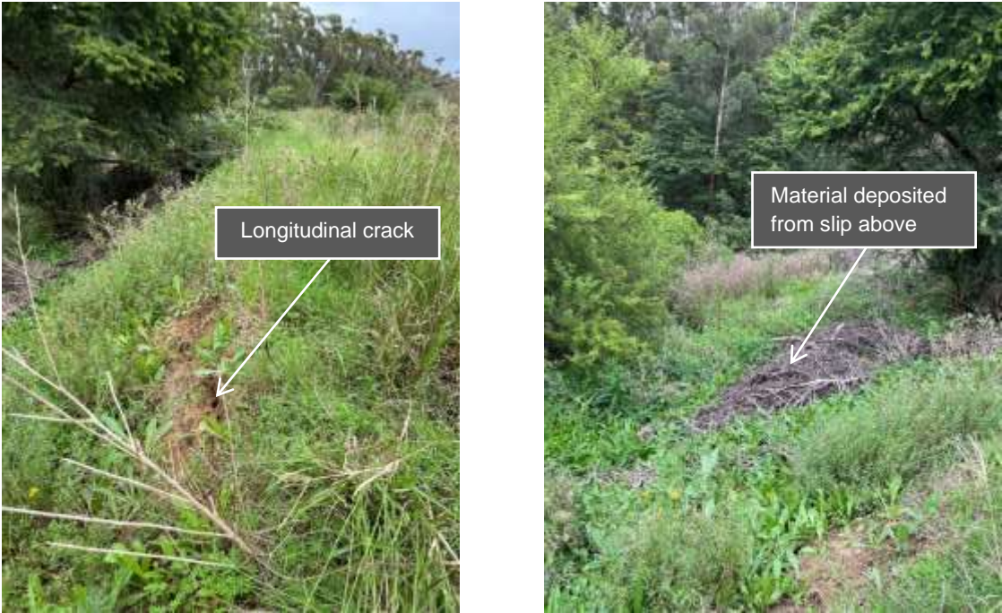
Figure 4-6: Steep sections caused by surface slips. Note thick vegetation and large trees on DS face.
