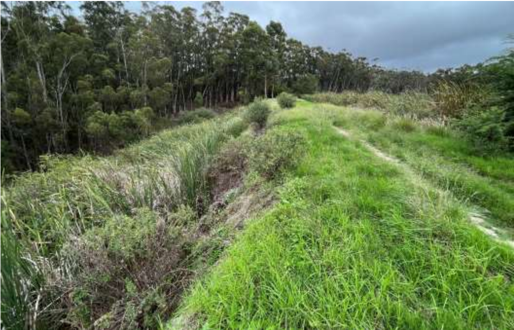
Figure 4-5: Surface slip near right abutment. Note reeds growing where seepage likely daylights.
