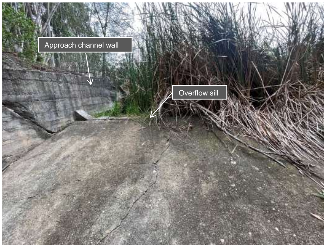
Figure 4-8: Looking upstream towards overflow sill. Note clogged with vegetation
