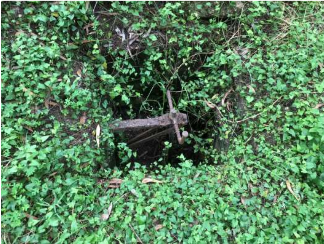
Figure 4-12: Spindle of suspected main outlet valve located at downstream toe of dam.
