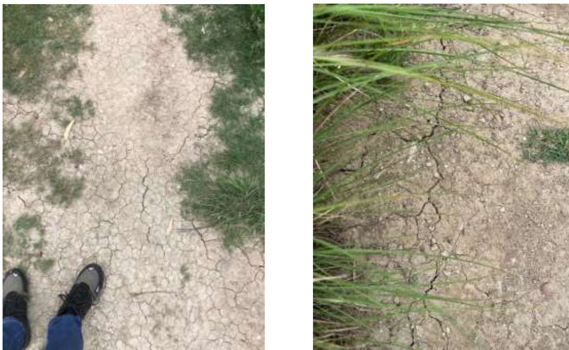
Figure 4-3: Desiccation cracks observed along length of the crest
