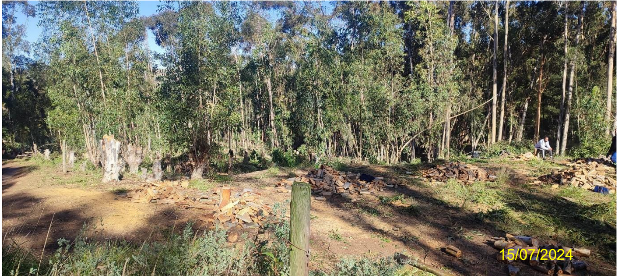
Photo 4: Eucalyptus tree clearing taking place on proposed development site below Bloekombos dam.
