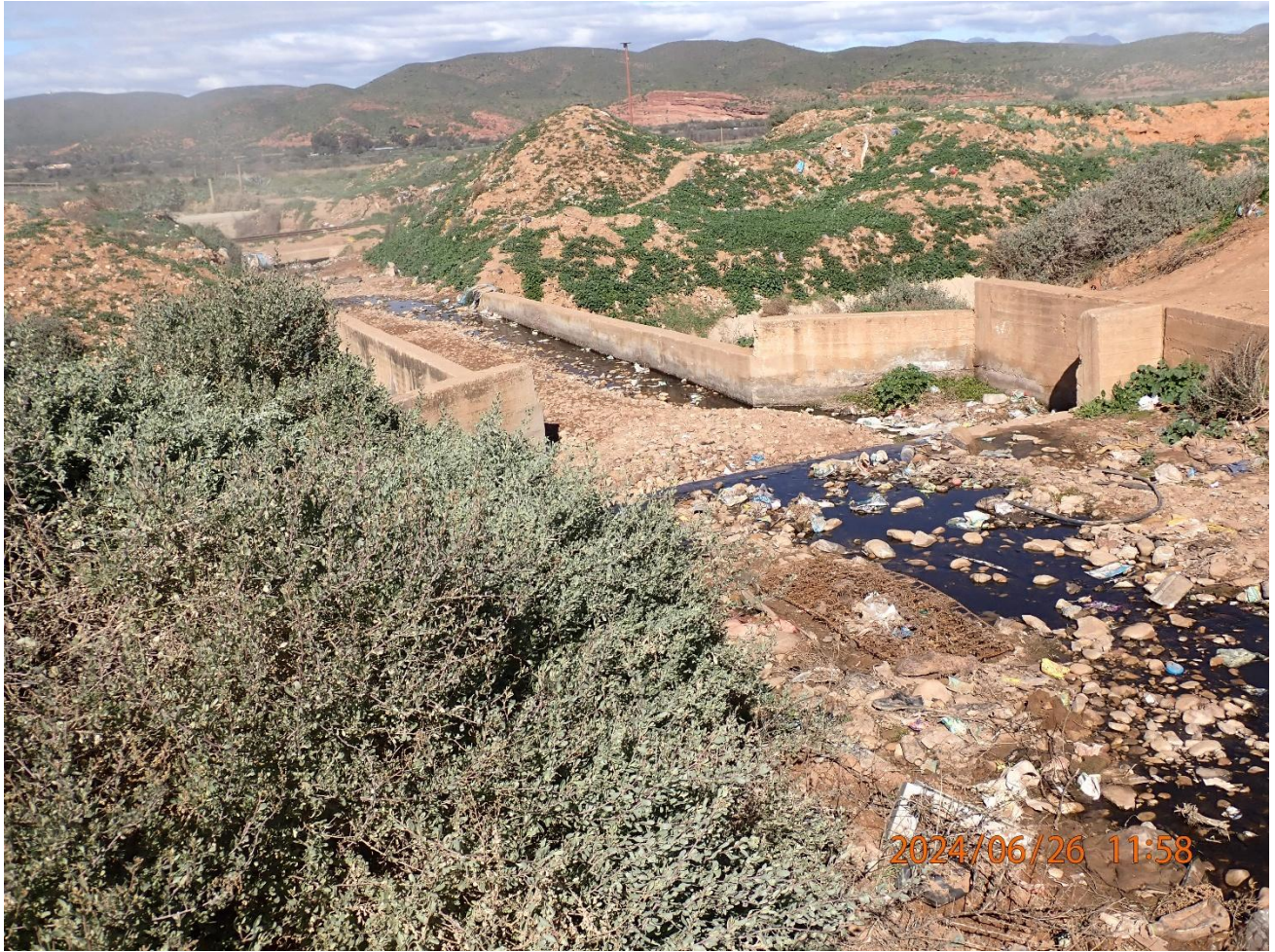
Photograph 20: Formalized downstream view of drainage line flowing underneath the road and irrigation water channel.
