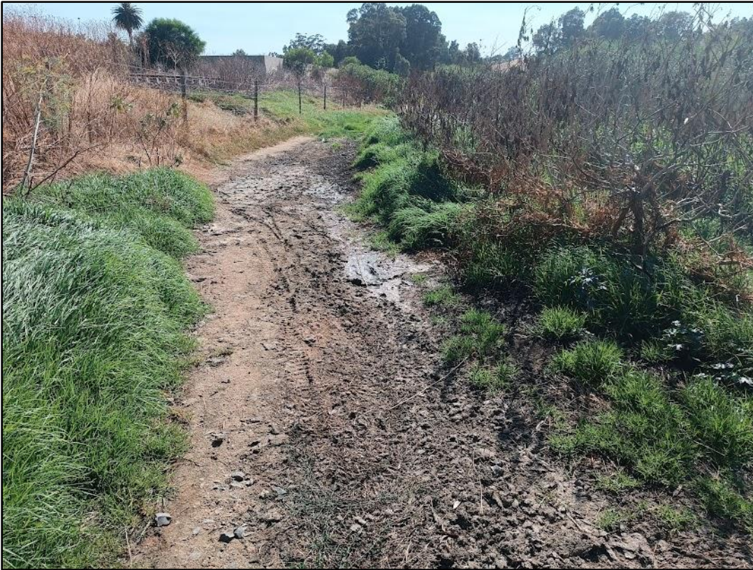
Figure 7: The area between the manhole and the Diep River showing signs of pollution from leakages from the manhole.
