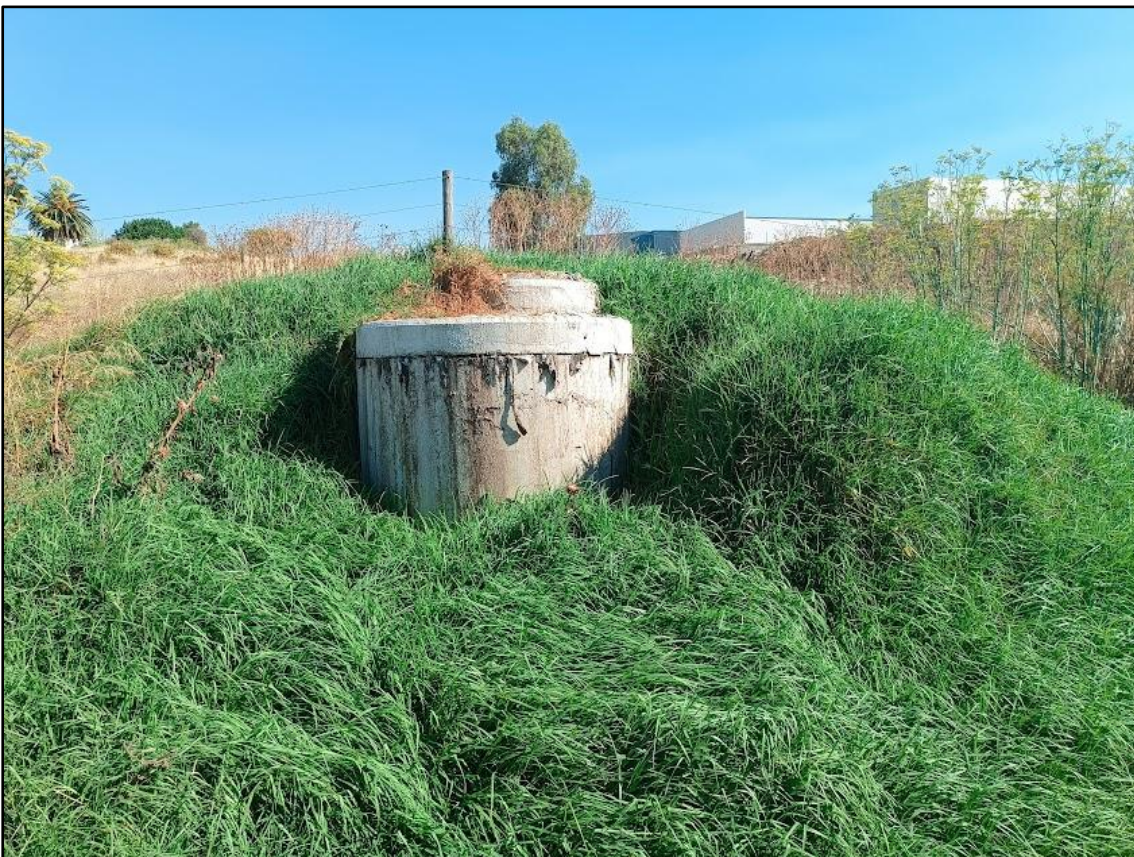
Figure 6: A manhole located immediately adjacent to the proposed pipeline crossing which shows signs of overtopping.
