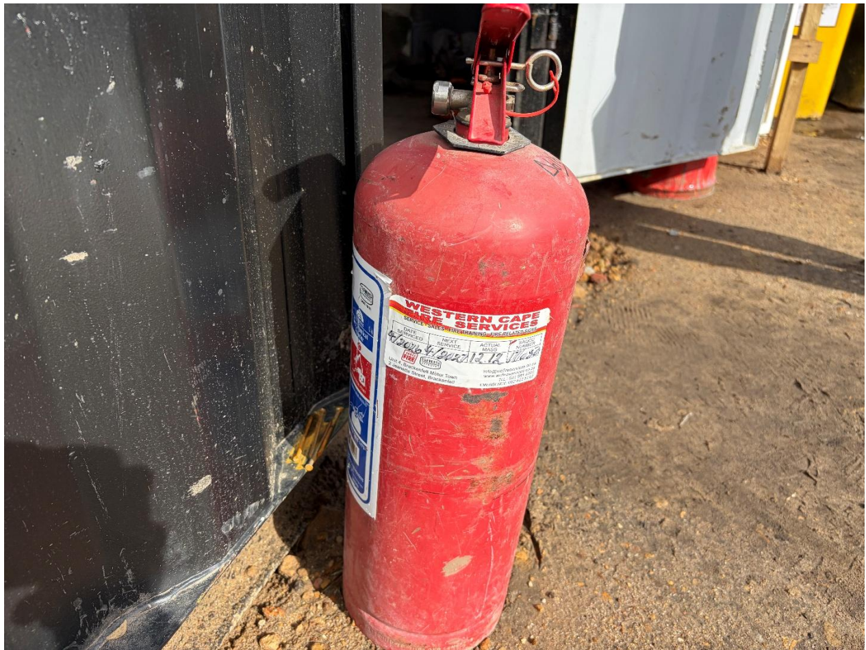
Photograph 9: Onsite firefighting equipment.
