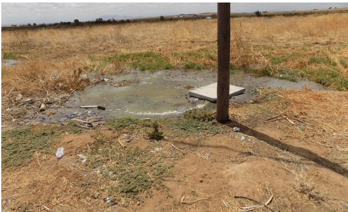
Figure 6.1. Raw sewage spilling directly into the surrounding environment.
